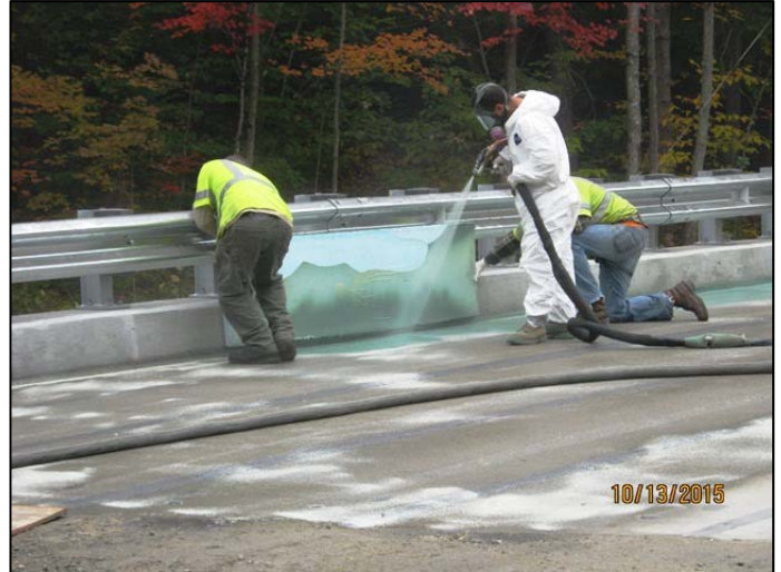
Sealing along the gutter line joint (between curb and slab) while masking the face of curb, sidewalk, and rail with plywood.
