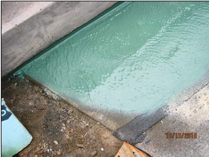
First course of Deckguard recently applied to the deck adjacent to the curb.
