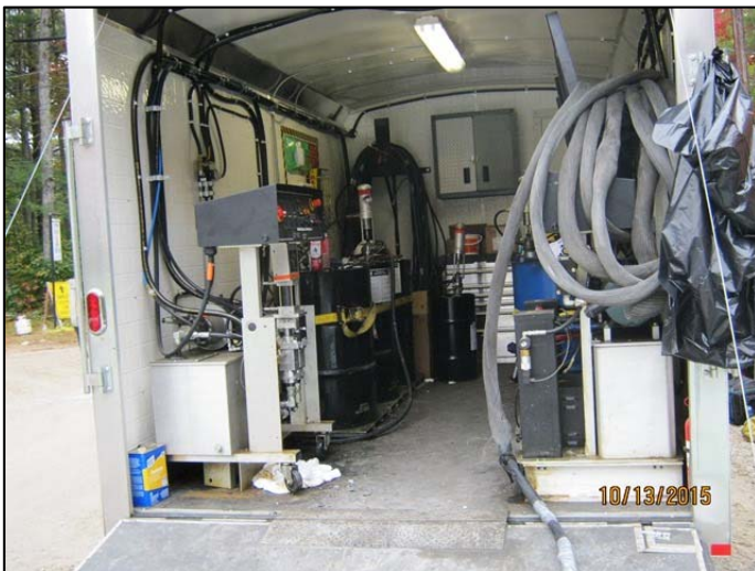
Deckguard Spray Membrane is spray applied using suitable plural spray equipment at a 1:1 mix ratio.
