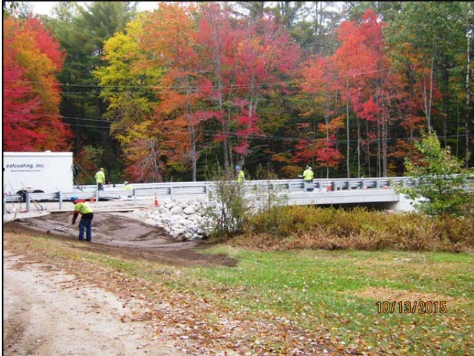
Prior to application, the deck was sandblasted, cleaned of any deleterious material, and primed. Ambient temperature was 60°F.
